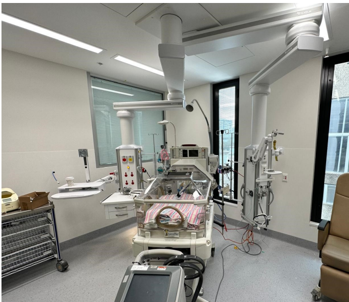
24 pendants will be installed boasting two arms
